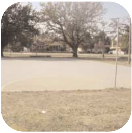
Before: the substandard surface
